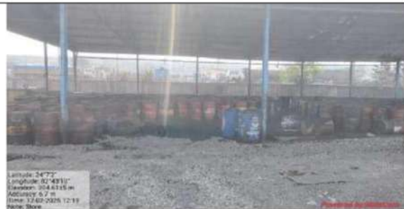
Pic 16 Cleaning of the spilled oil during lifting with all burnt oil under shed.
